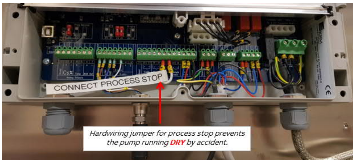
Figure 1. Process stop jumper wiring of delivered white water sensor with pump.
