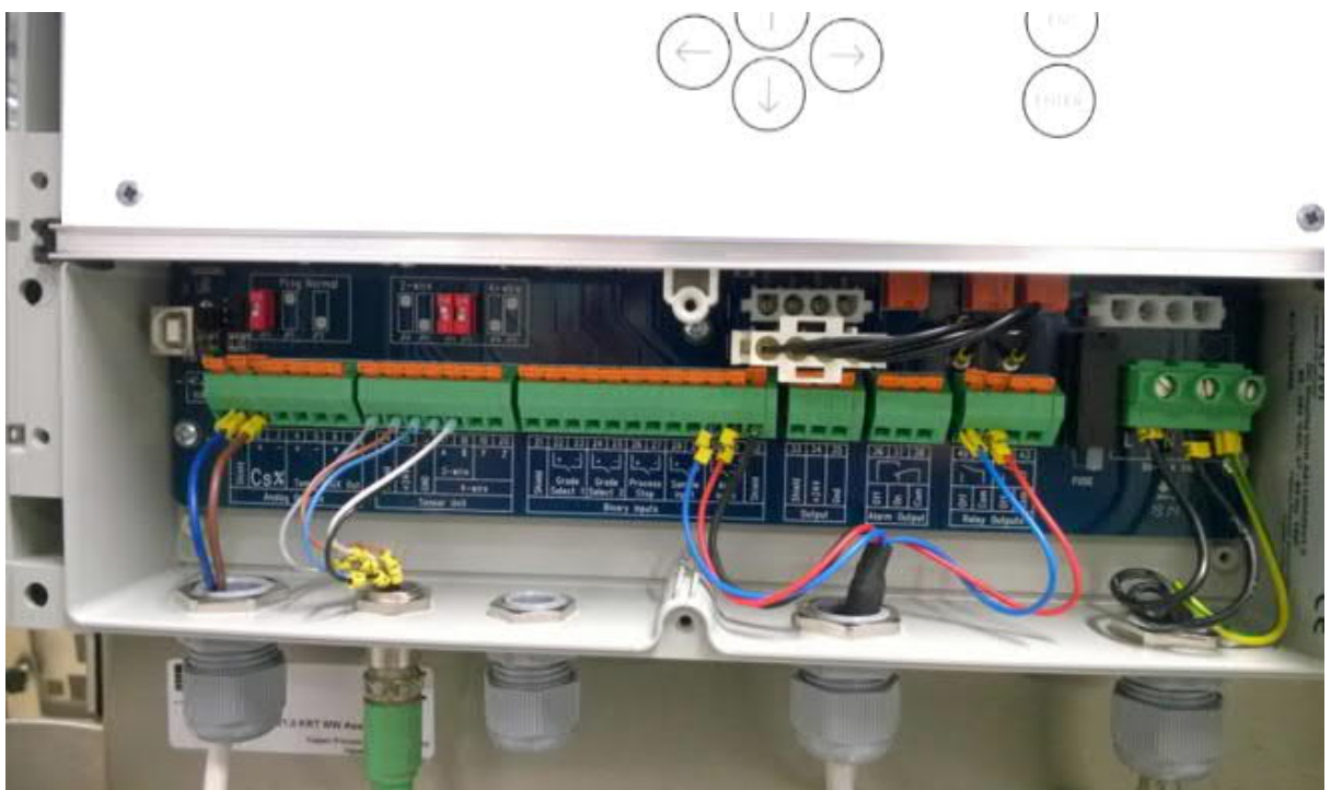
Figure 11. KC9 Display unit wiring.
