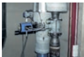
Oden P50R - "Hot water control" District heating plant, Tekniska verken, Linköping, Sweden
